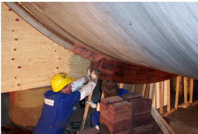
Bonding of dehonit® / Perмали fixed bearings under the world's first LNG cylinder Tank
